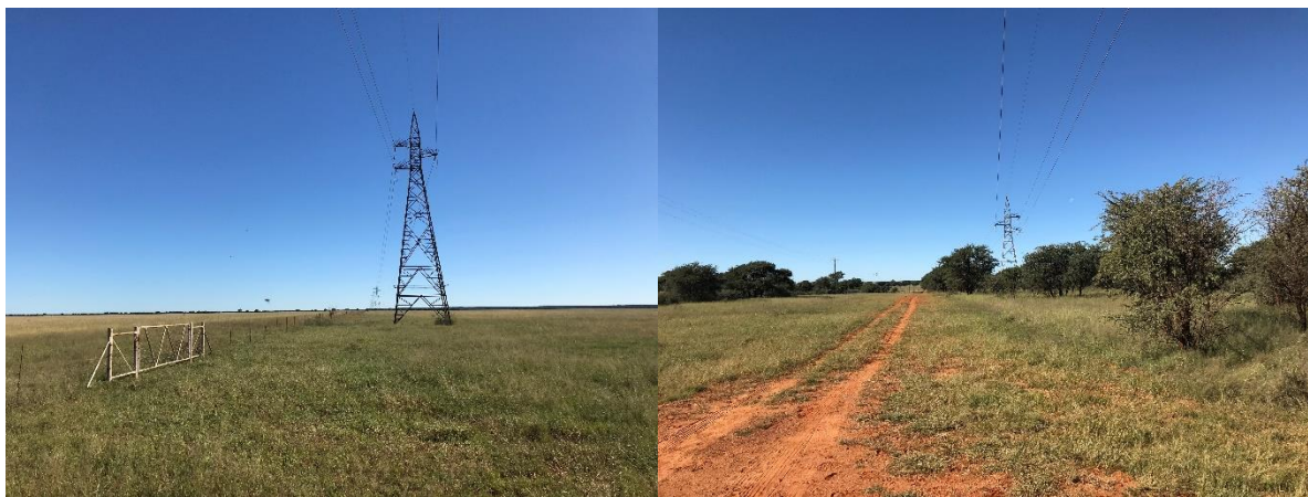
An existing overhead powerline that is associated with Option 2 for a short distance.
